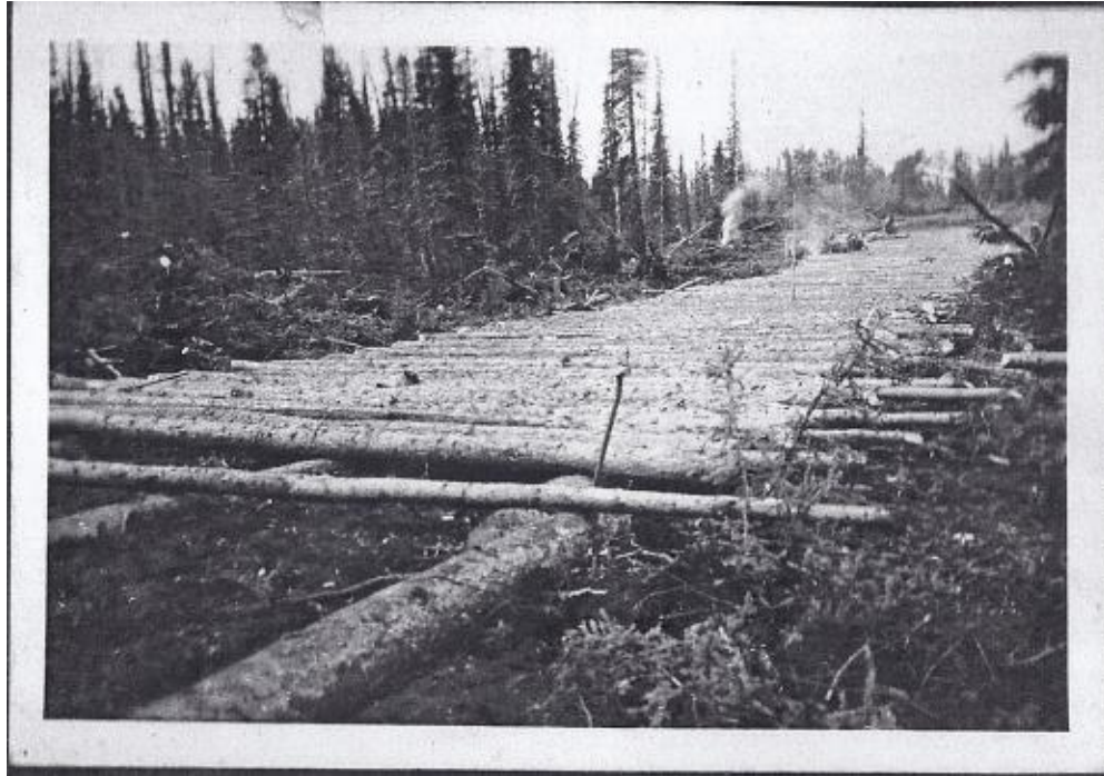
Image 4.4 Corduroy road construction along the Alaska Highway. Yukon Archives, Andrew Porubsky Fonds 2007/7 PHO 636#30084
