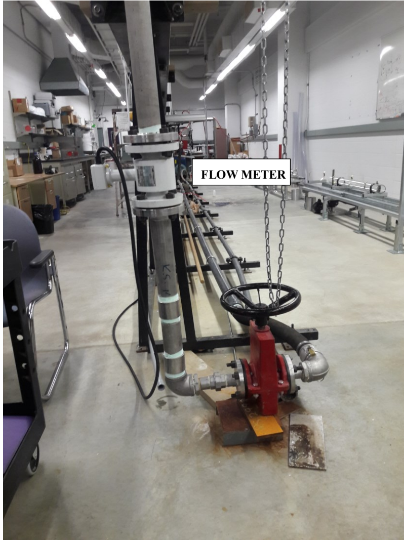
Figure 2-6 The magnetic flow meter in the horizontal loop.
