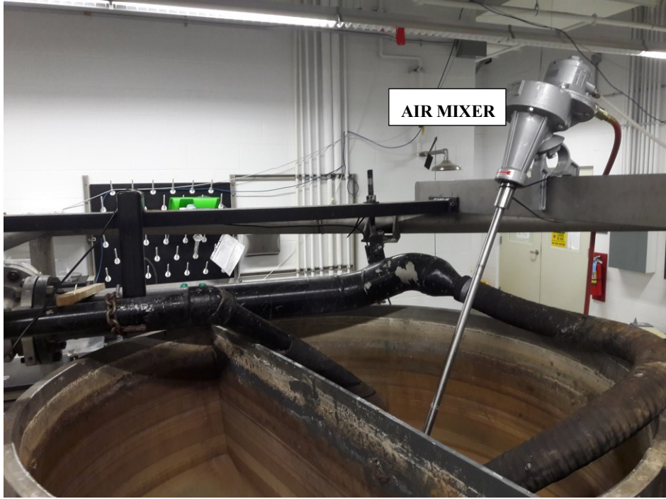
Figure 2-3 The air mixer installed on the suction tank.
