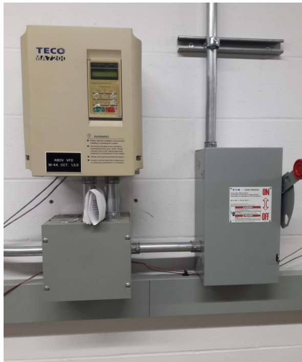
Figure 2-4 VFD unit controlling the electric motor.
