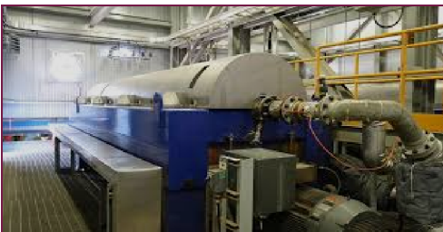
A tailings centrifuge unit in at Albian's Jackpine Mine.
