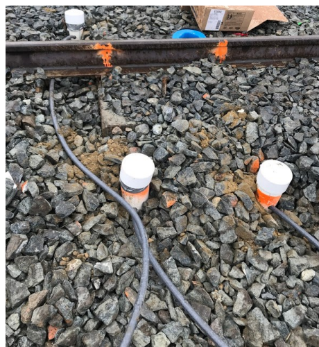
Figure 3.18. Protection of wires using PVC electrical conduit on May 15, 2019 (Abdulrazagh 2019 – with permission).
