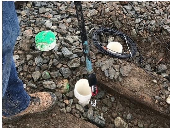
Figure 3.17. 5TE sensors installation using a notched pipe on May 15, 2019 (Abdulrazagh 2019 – with permission).
