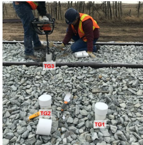
Figure 3.15. Installation of access pipes in the track on April 24, 2019 (Abdulrazagh 2019 – with permission).
