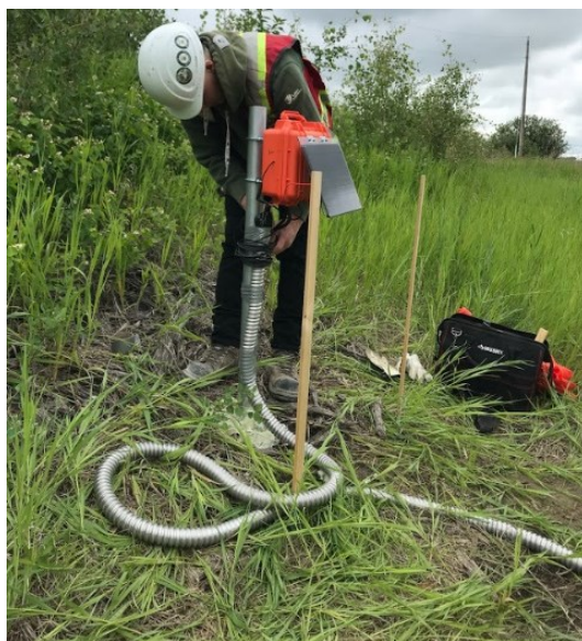
Figure 3.19 - Protection of wires by metal electrical conduits where the cables could not be buried beneath the soil on May 15, 2019 (Abdulrazagh 2019 – with permission).
