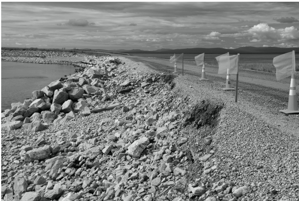
Figure 3. The Nome-Council Highway View of erosion and road collapse. Photo was taken by author during the summer.
