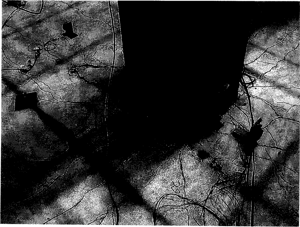
Figure 4.39 (a) Crack Pattern of Sp-A after Failure
