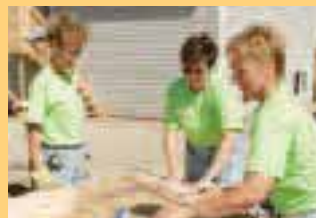
PotashCorp volunteers help construct a home during an August 2004 Habitat for Humanity event.
