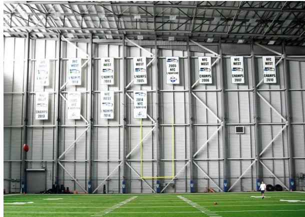
Figure A.1: Five-tiered BRBFs used in the Seattle Seahawks indoor practice facility in Renton WA (Courtesy of Michael Lawrie).
