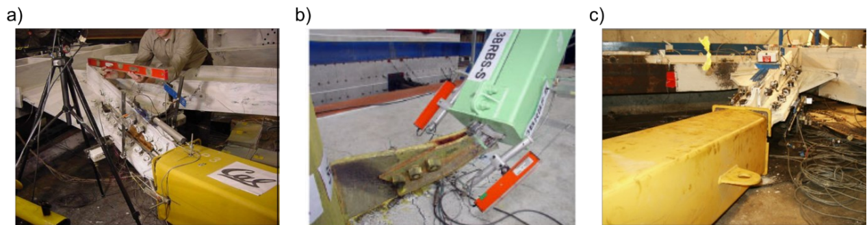
Figure 2.5: BRBF connection failures: a) Uriz and Mahin 2005; b) Tsai et al. 2008; c) Palmer et al. 2014.
