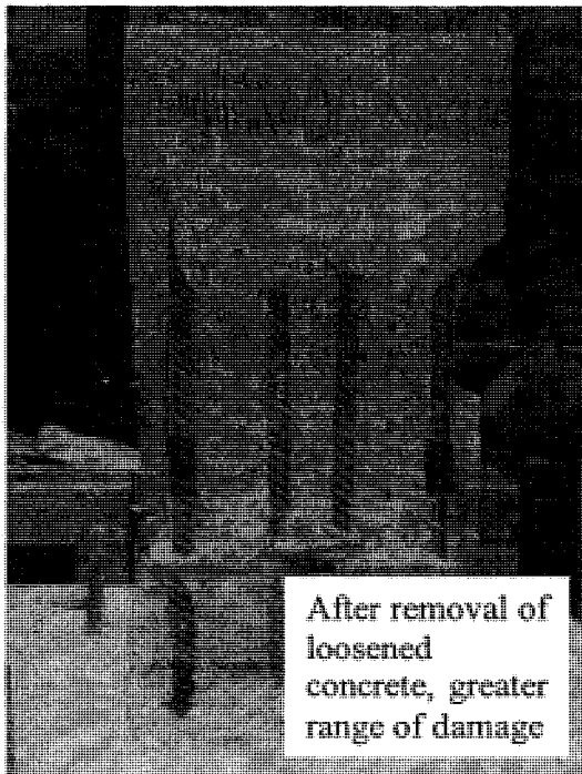
(c) At end of test (North side)
