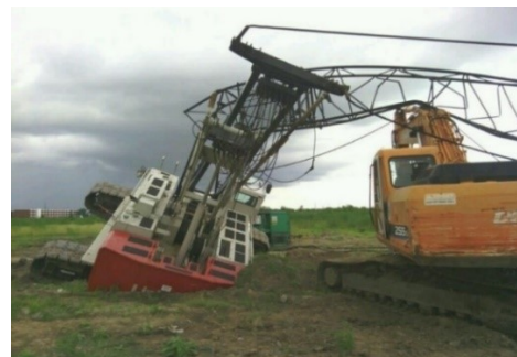
Fig. 1-2: Soil collapses under crane load
