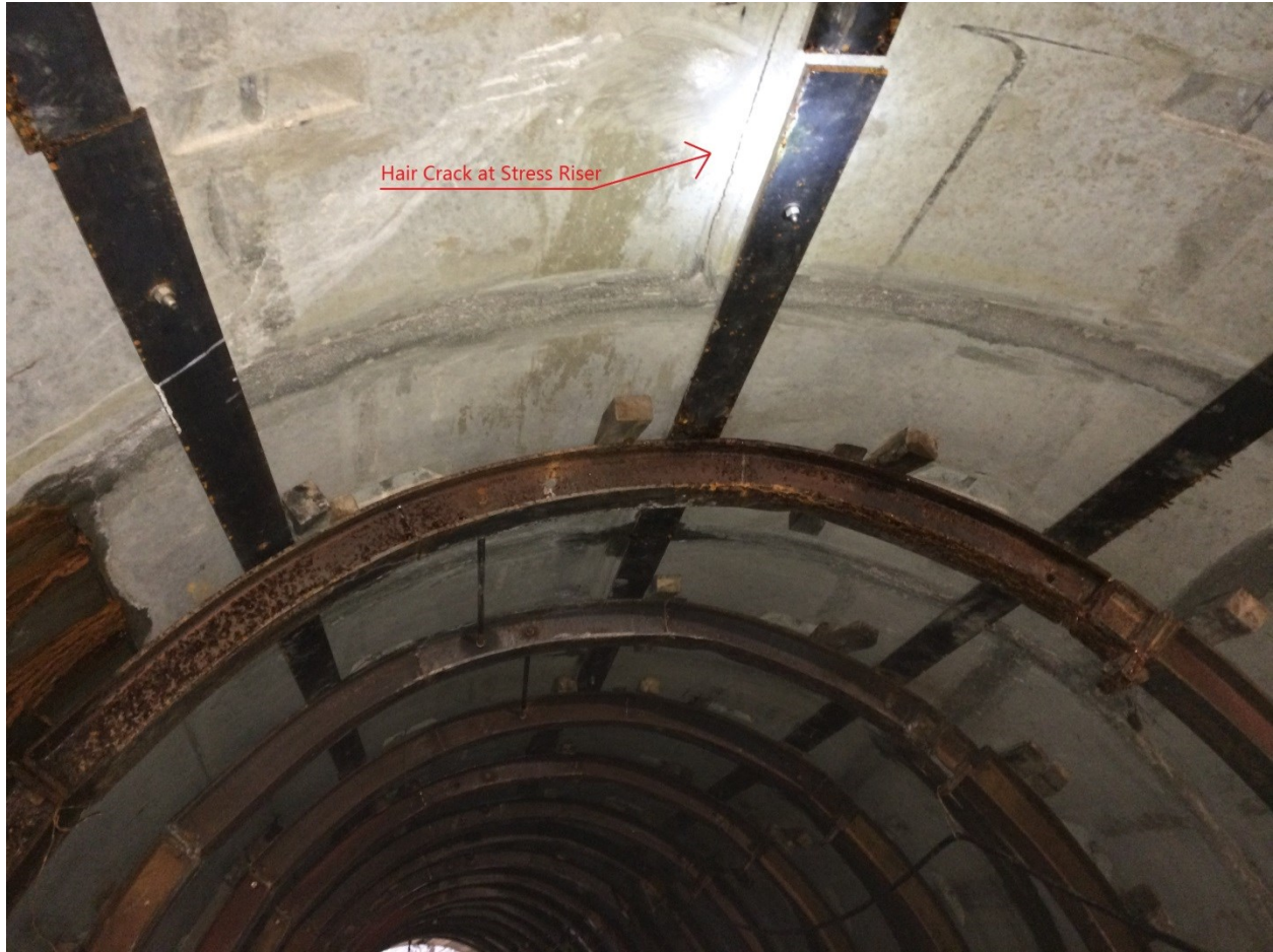
Figure 6-5 Hair Crack at Stress Riser and Reinforcements (Circular Steel Ribs and Straps) Installed
