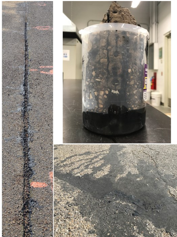
Figure 5-6: Distresses encountered in the aggregate + emulsion segment (I-J)
