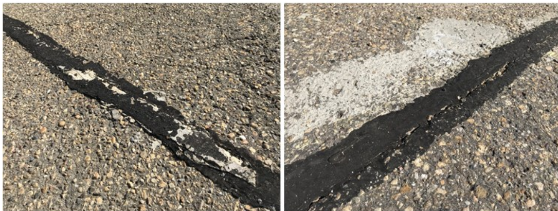
Figure 5-5: Distresses encountered in grout + sealant segments. (a) F-G. (b) H-I
