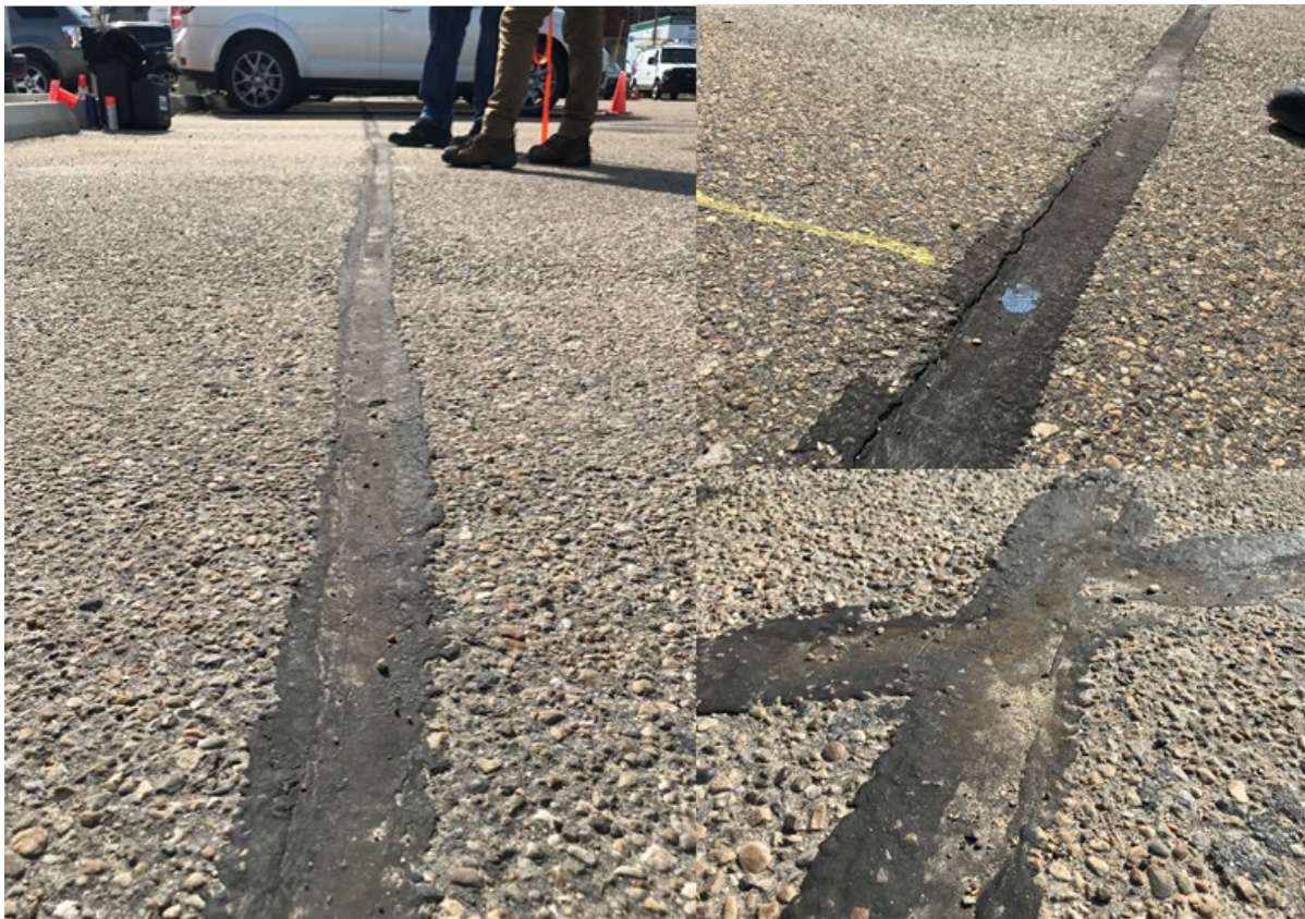
Figure 5-7: Distresses encountered in the grout + cold mix + sealant segment (A-F)
