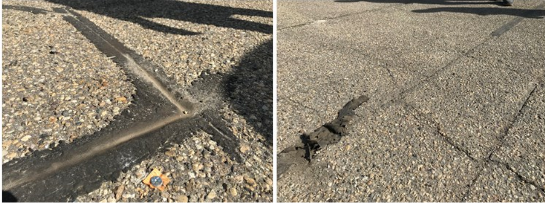
Figure 5-4: Distresses encountered in SMCI segment
