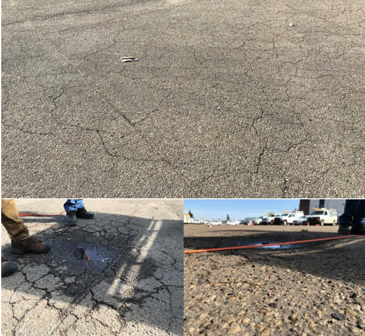
Figure 5-3: Distresses encountered in VIF segment
