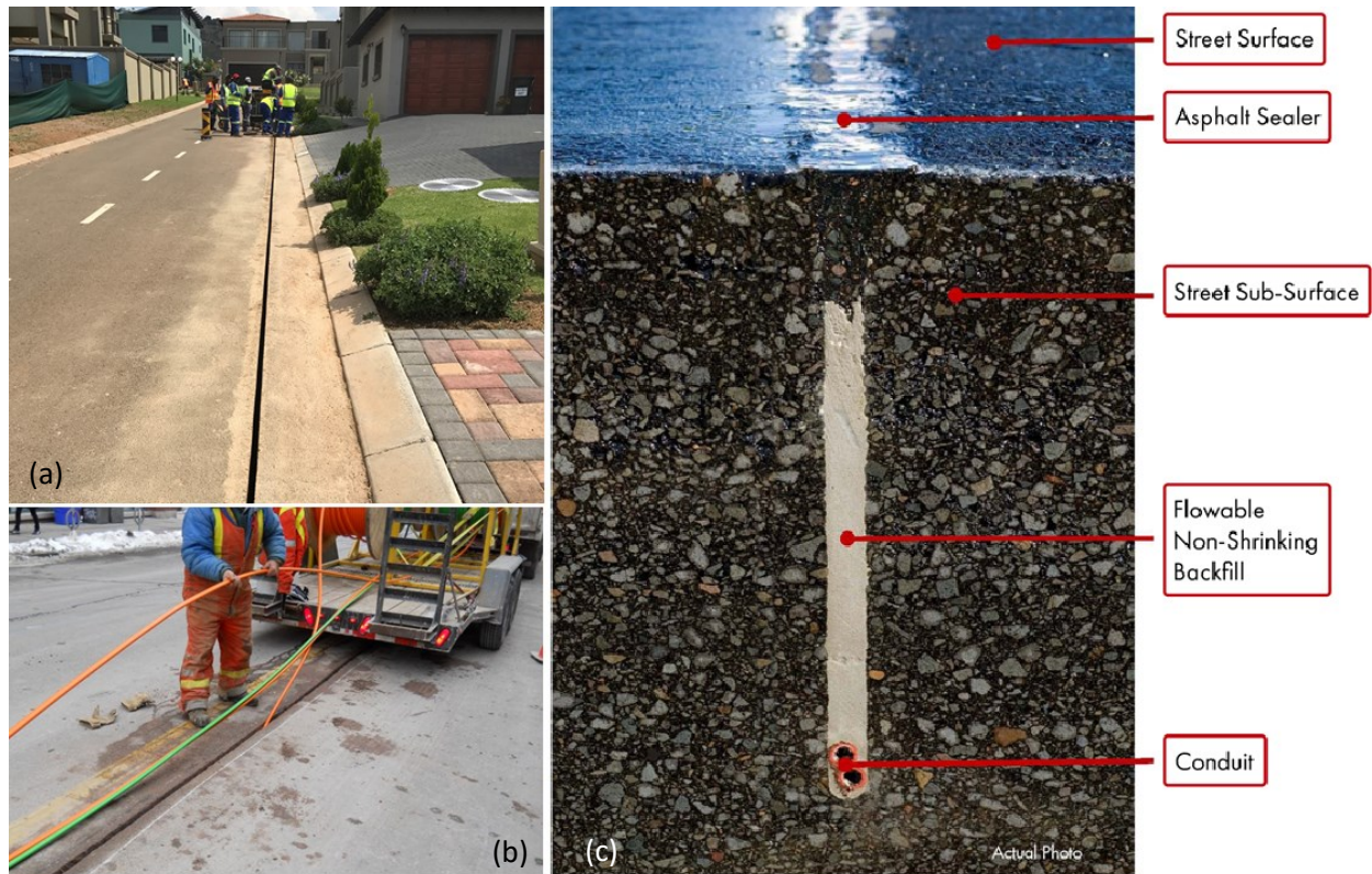
Figure 2-1: Micro-trenching application. (a) Cutting (Linteg Technologies). (b) Laying cables (The Fiber Optic Association). (c) Backfill cross-section (Certus View)
