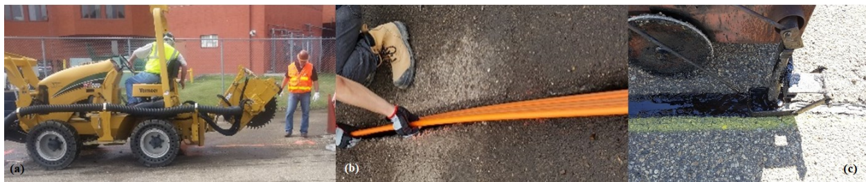
Figure 3-1: Micro-trenching procedure (Rezai, 2016). (a) Cutting the trench. (b) Laying cable. (c) Backfilling
