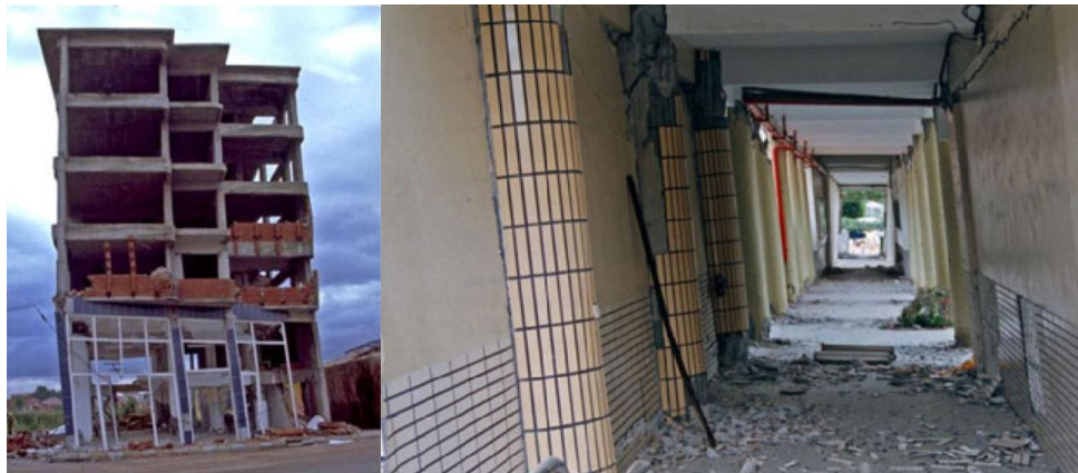
Figure 2.1. ‘Examples of buildings with residual displacements leading that typically lead to demolition (left photo by M. Bruneau, MCEER; right photo by A. Whittaker, NISEE, EERC, UC Berkeley)’ (Ramirez and Miranda 2012)
