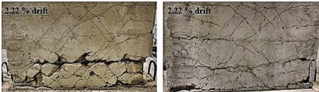
Figure 2.24. Damaged state of specimens (Ghazizadeh 2017)
