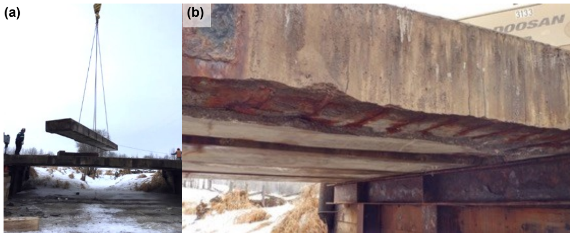
Figure 3- 6: (a) Bridge being taken apart, (b) photo of heavily deteriorated girder.
