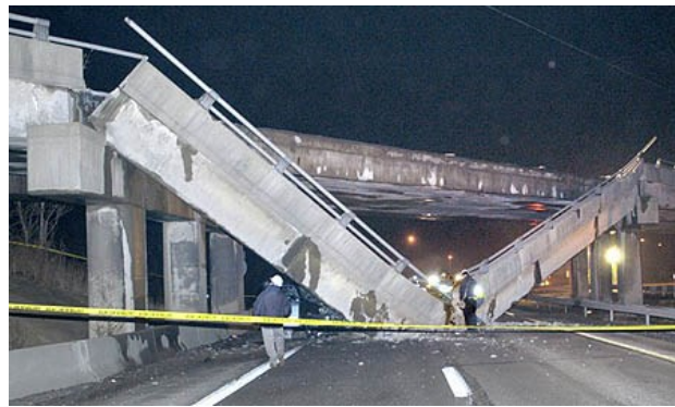
Figure 2- 5: Collapse of Lake View Drive bridge girder in 2005 (Panchak, 2005).
