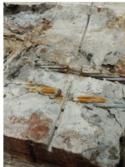
Figure 3- 10: Induced (cut) strands loss in Girder ID.
