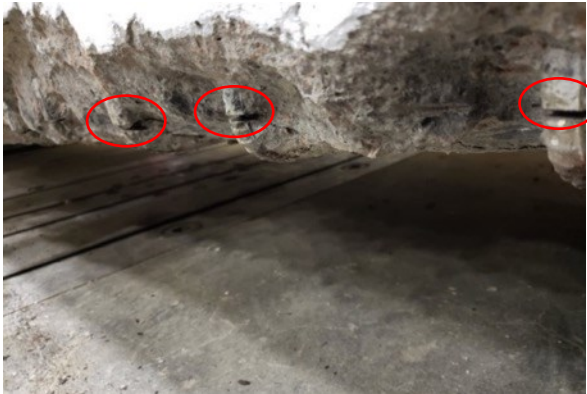
Figure 4- 15: Cut stirrups (cuts circled) on girder MD-1.5S. These stirrups had limited deterioration as evidenced by their colour and lack of pitting corrosion.
