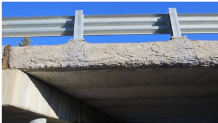
Figure 3- 2: Concrete section loss due to freeze and thaw damage (AT, 2017).
