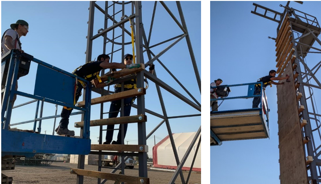
Figure 4.19: Wood backing system to support airbag (a) Installation of wood joists (b) Installation of plywood sheets.
