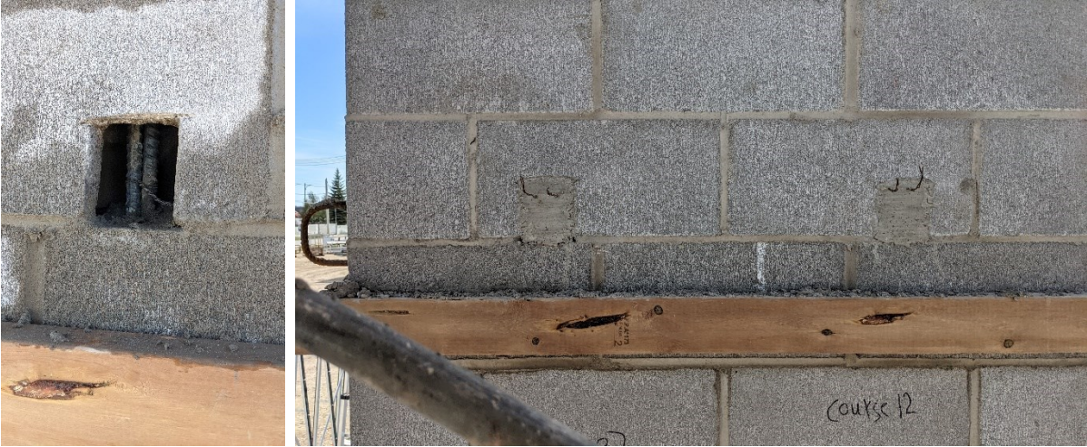
Figure 4.5: Cleanouts as required by A371 (a) Before grouting (b) After grout hardened.
