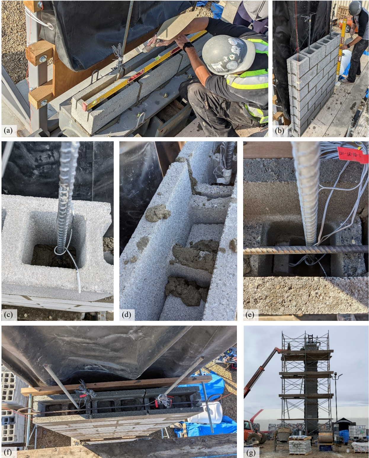
Figure 4.6: Construction process for the masonry wall (a) Certified mason laying the first course (b) Mason checking the verticality of the wall (c) Use of positioners to secure position of bars (d) Blocking void cells to prevent grout from entering before grouting a bond beam (e) Horizontal reinforcement in bond beam (f) Construction progress view from scaffolding (g) Scaffolding used to build the masonry wall.
