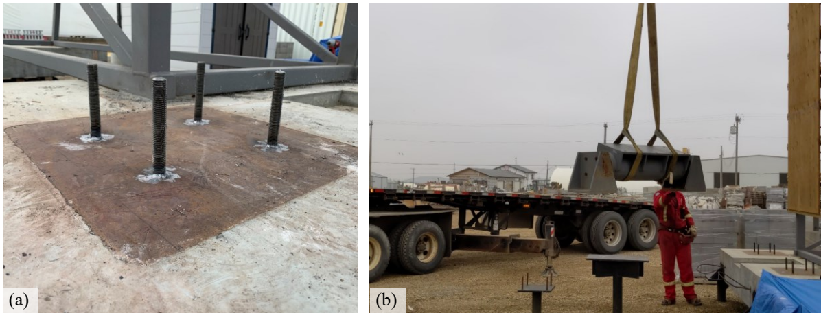
Figure 4.17: Rotational base installation (a) Threaded rods welded to the plates on the slabs (b) Device lifted by a crane to install on top of slab.
