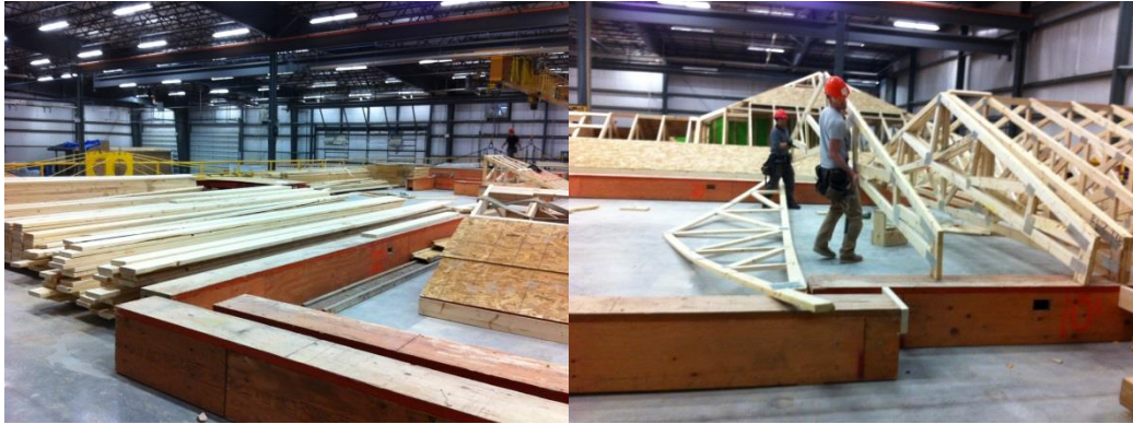
Figure 63: Roof station deficiencies
