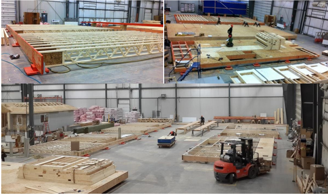
Figure 60: Floor station after implementation of proposed improvement
