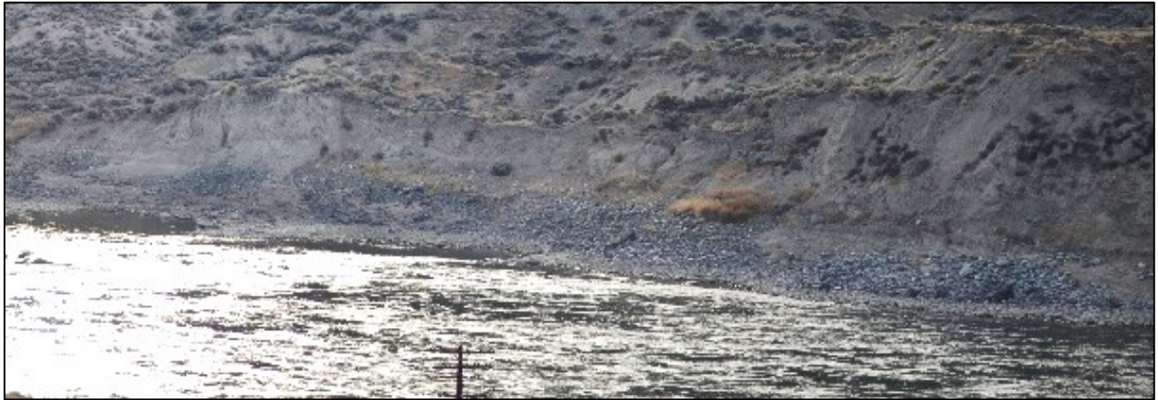
Figure 5-10: Active Erosion and Sloughing of the Red Hill Toe (looking southwest)
