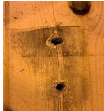
(f) Wood splitting around panel joint.
