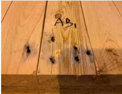
(e) Wood splitting around base shear connections and panel edge tear out.
