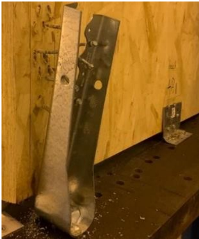
(a) Screws withdrawal; deformation of hold-down.
