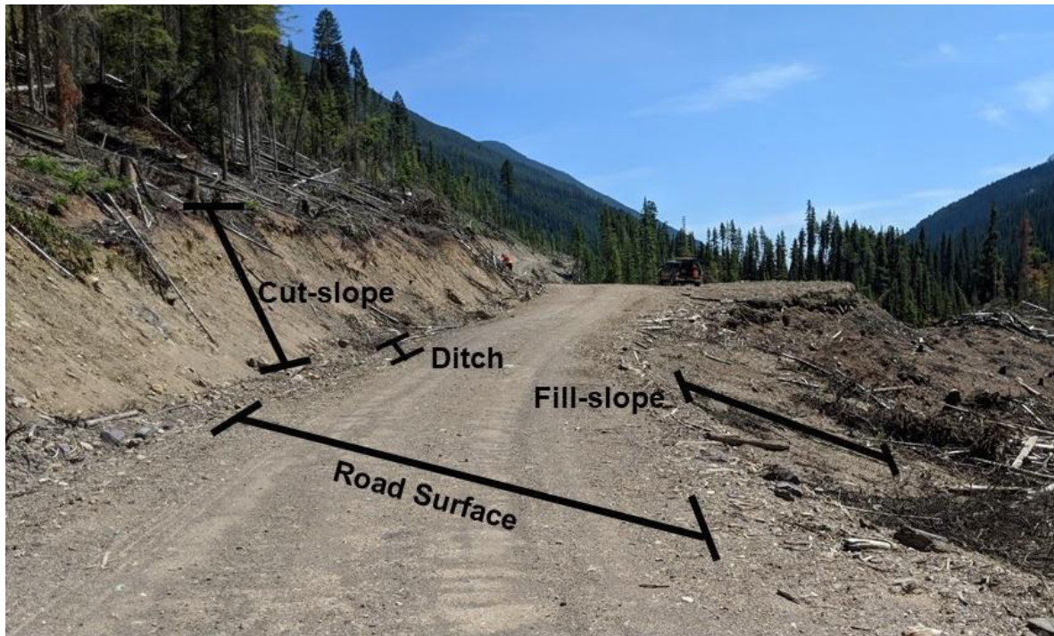
Figure 2-2 Road build diagram. An unpaved road generally consists of a road surface that can be crowned and a ditch. Roads on hillslopes will have cut and fill slopes.
