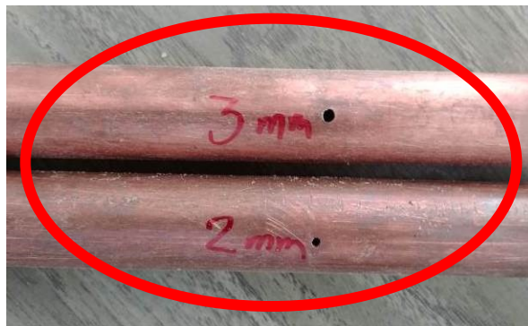
Figure 4.17: Small leak source (Pinholes)
