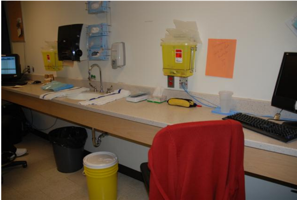
Figure 5-2: Water splashing on side of sink (C-MG-59)
