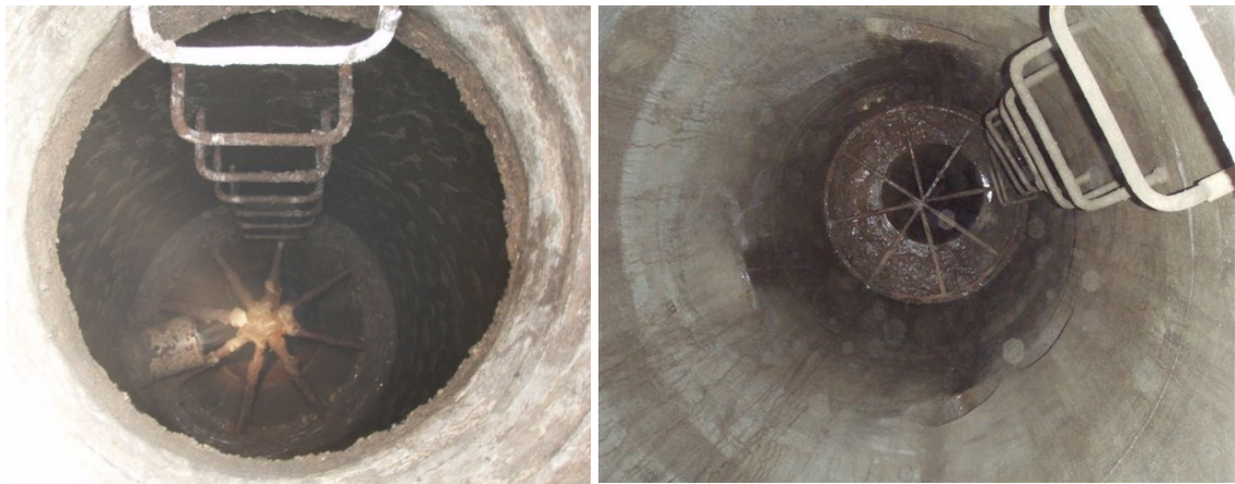
Fig. 1.1 Pictures of Drill Drop Manhole (DDM) in city of Edmonton, photo from Smith (2013)
