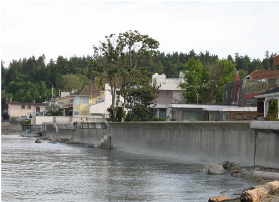
Figure 10 Photo highlighting variations or “lips” at the tops of the seawalls
