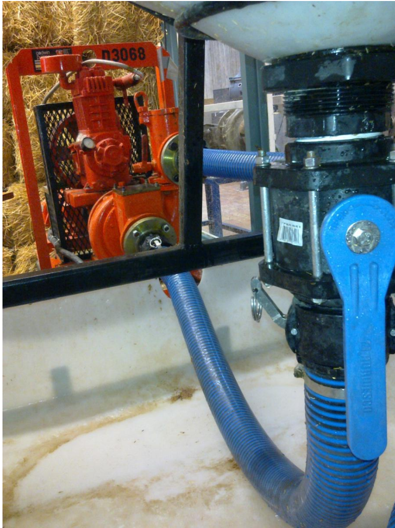
Figure 27: Hose bend in wide radius connects the pump to mixing tank
