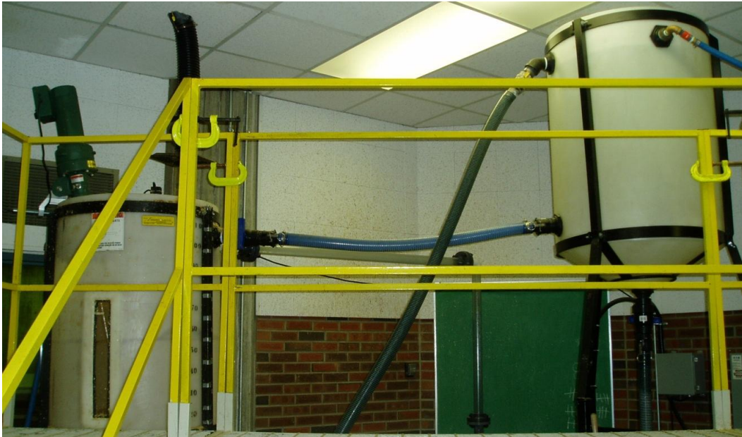
Figure 30: The dilution tank is elevated above the mixing tank
