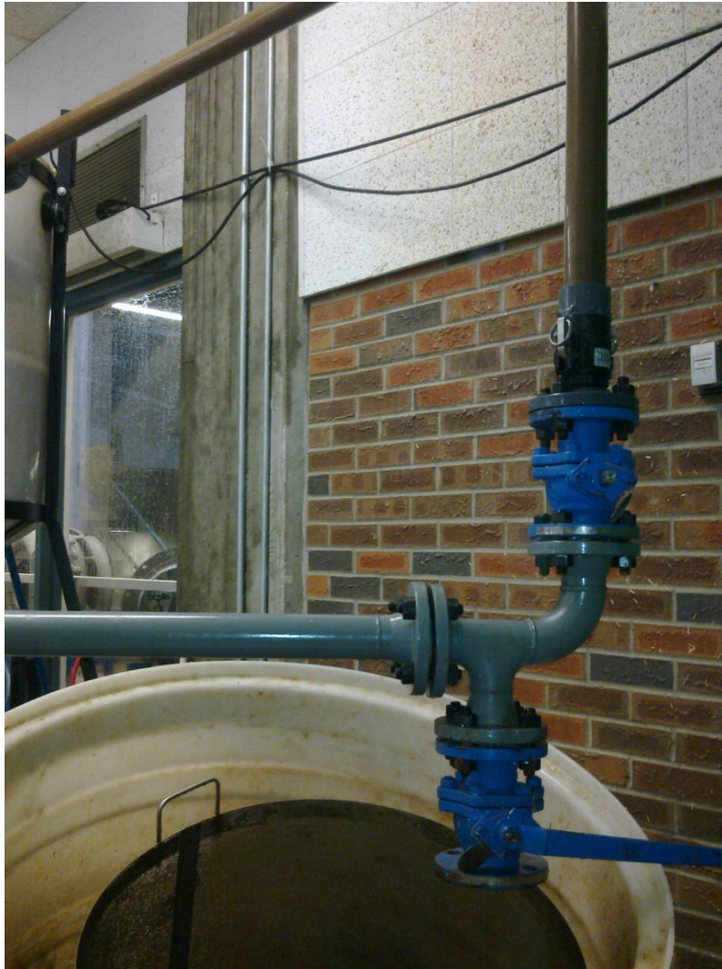
Figure 31: Transparent PVC return line links discharge valve to mixing tank
