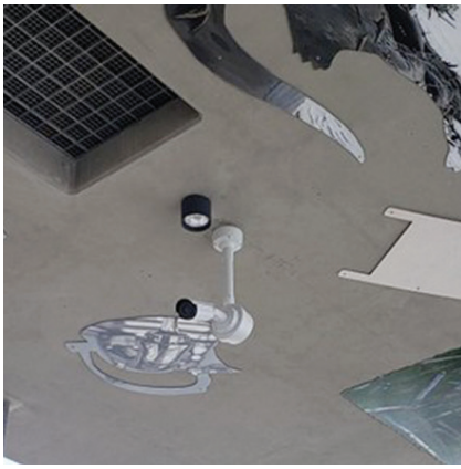
FIGURE 4a: Security Camera on bridge deck (1 of 2) [Quecke, E. April 2, 2023]
