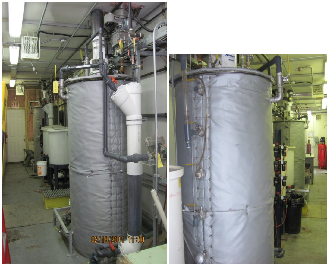
Figure A2. Pilot Anaerobic Digesters
