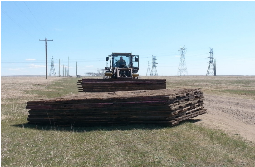
Figure 3-2. Access matting transmission tower construction where access mats (bottom) were used to build access trails into the tower sites (top), as well as establish a working area directly below the tower to facilitate tower assembly and erection.
