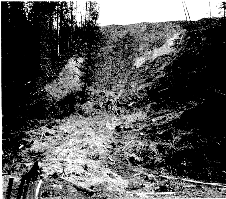
Figure 14 Morkill 31.5 km (Figure 2): Earth slide in sandy soil below an abandoned cutting permit access road
