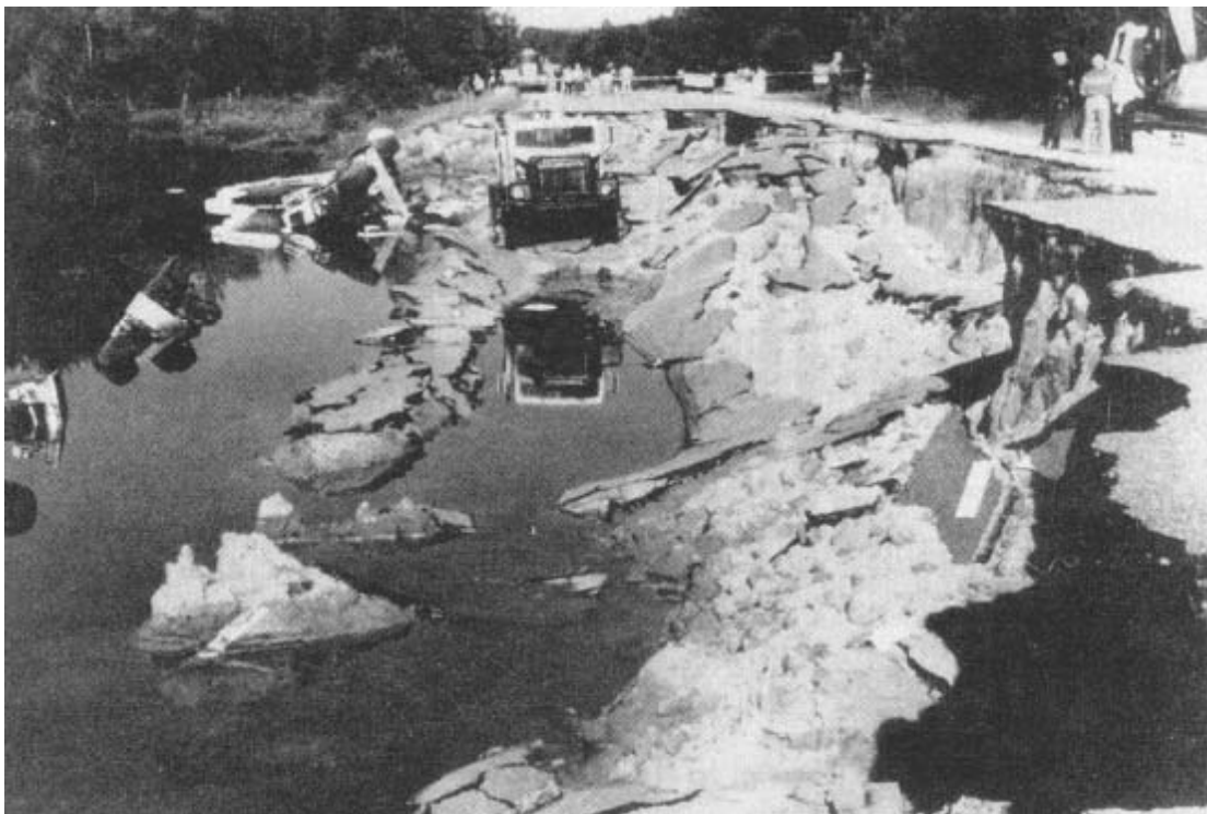
Figure B.32 Failure of the embankment on Ackerman Lake (After Hryciw et al. 1990)
