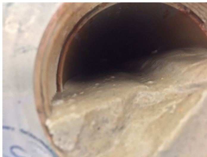
Figure 4.4: Slurry blockage of the pump supply line
