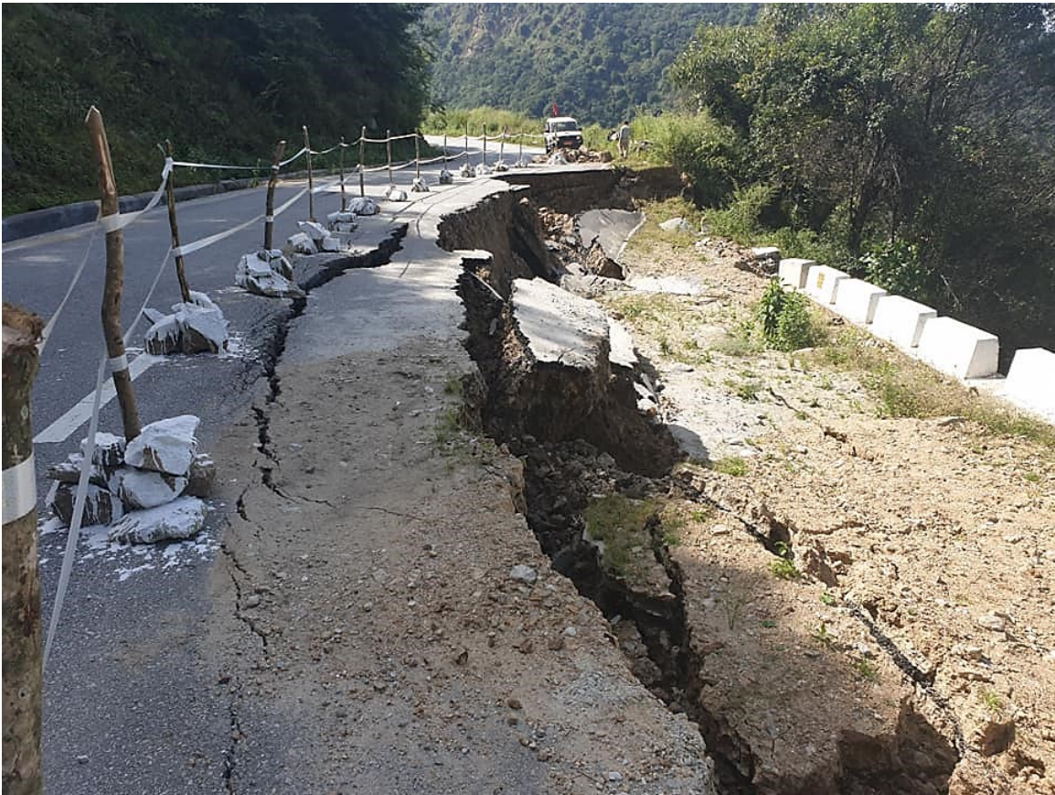
Roadblock due to subsidence/landslide
