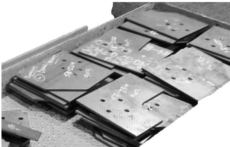
Figure 3-6: Cut plates with drilled holes ready to be welded to steel sections
