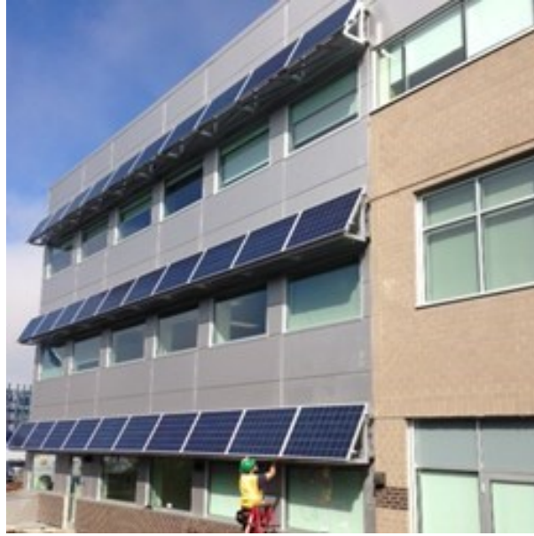
Figure 23: Wall-mounted solar PV panels at Landmark Business Centre
