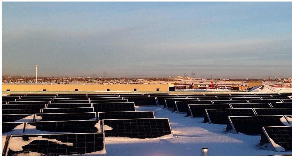
Figure 24: Rooftop solar PV system at Landmark Business Centre
