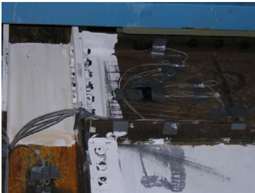
(f) North top connection, Cycle 18-Unload
