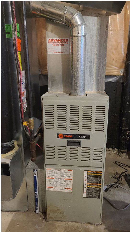
(a) Gas furnace
