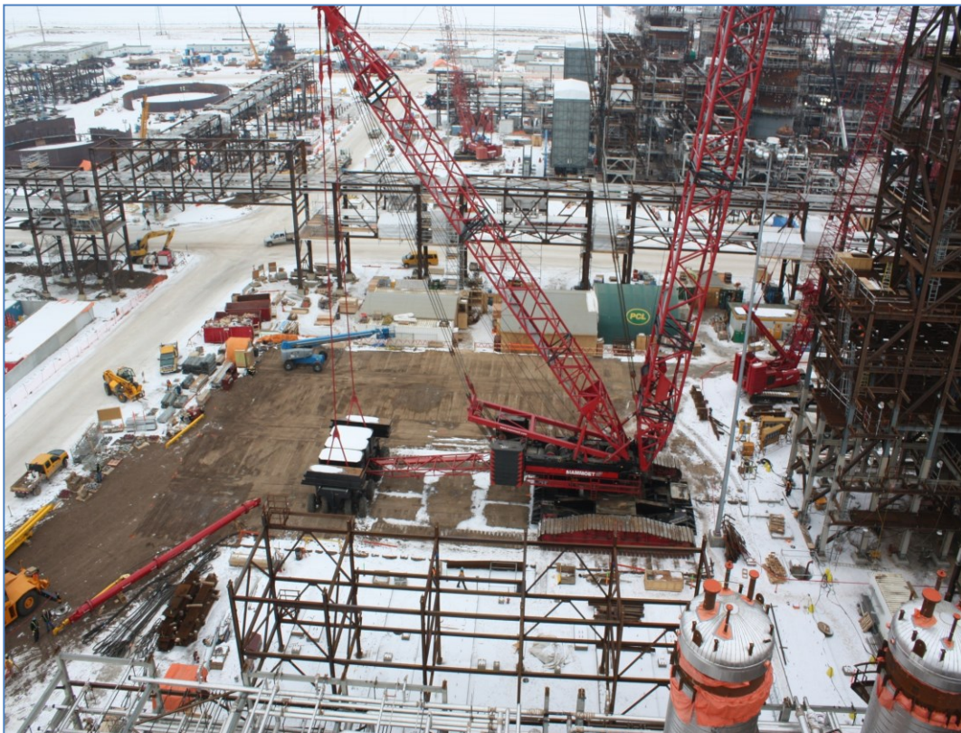
Figure 1-3 Typical industrial installation site
