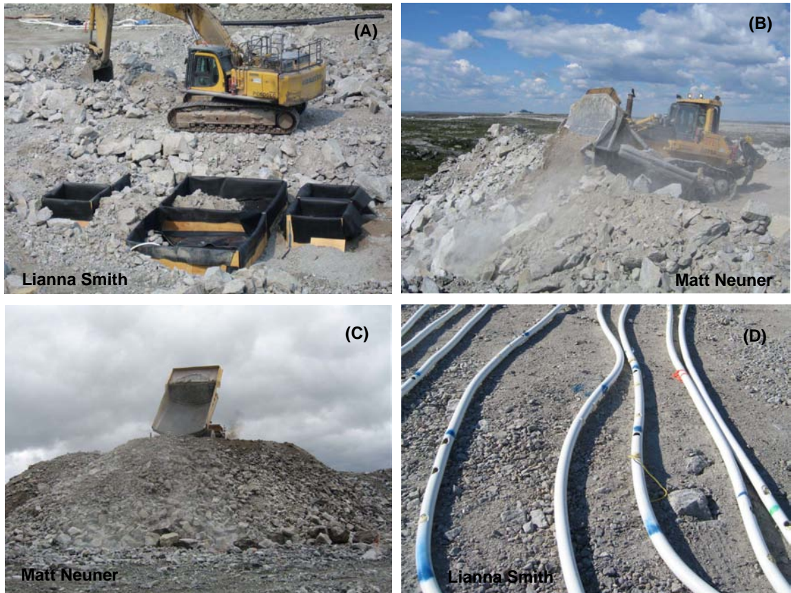
Figure C.15: (A) Basal lysimeters, (B) Push-dumping, (C) End-dumping and (D) thermistor cables are housed by flexible PVC tubings for protection during the replacement of waste rock
