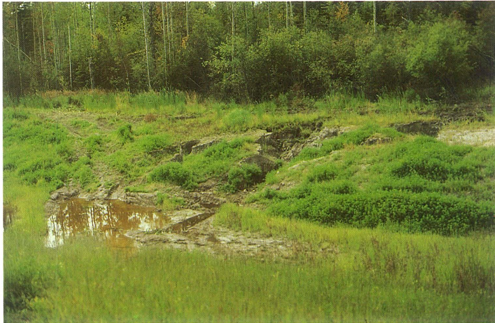
PLATE 5. Heavy silting at a gully formed by erosion along the West Interceptor Ditch.
