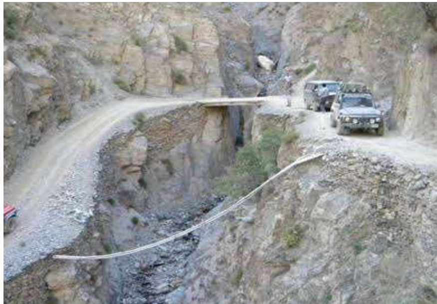
Figure 4. Unstable roads in the mountainous region of Chitral
