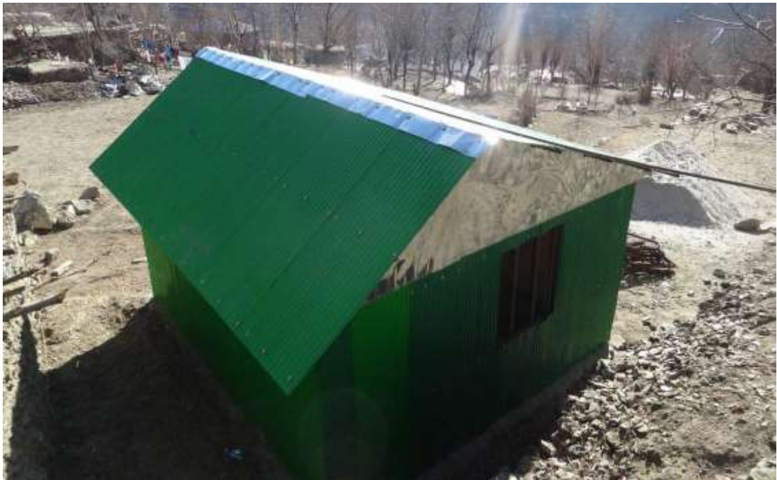
Figure 8. Angle iron model of the green shelter constructed and allocated by the Aga Khan Agency for Habitat to the 415 flood-affected families in Chitral during 2015-2016
