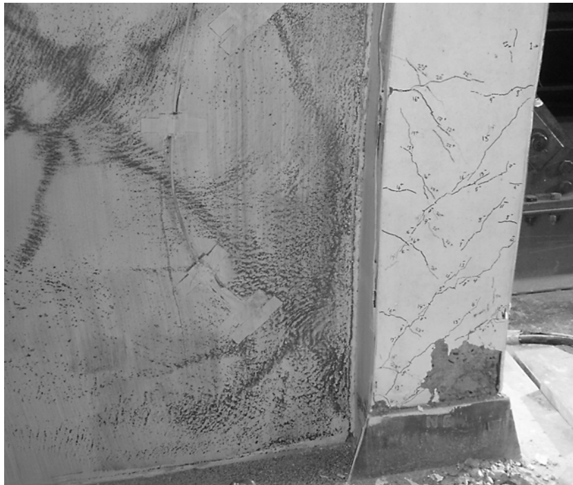
Figure 6.12: Base of the north column and adjacent infill plate at the end of the test
