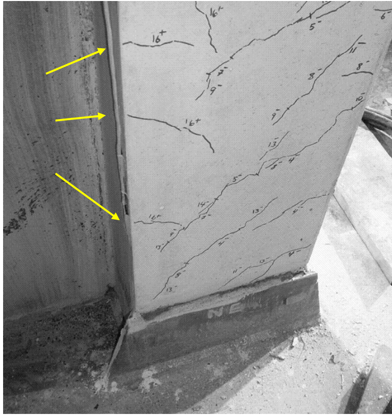
Figure 6.26: Base of north column in cycle 16 + and initiation of new cracks, adjacent to the inner flange of column
