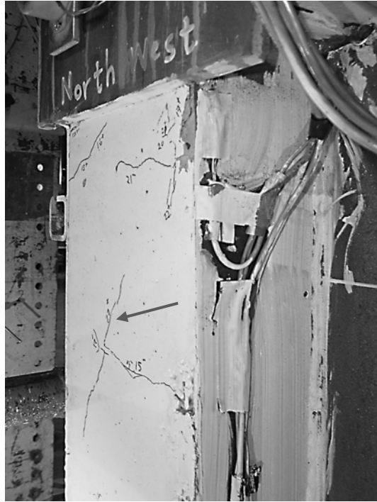
Figure 6.5: Diagonal crack close to top of the north column on west side in the first story during cycle 22
