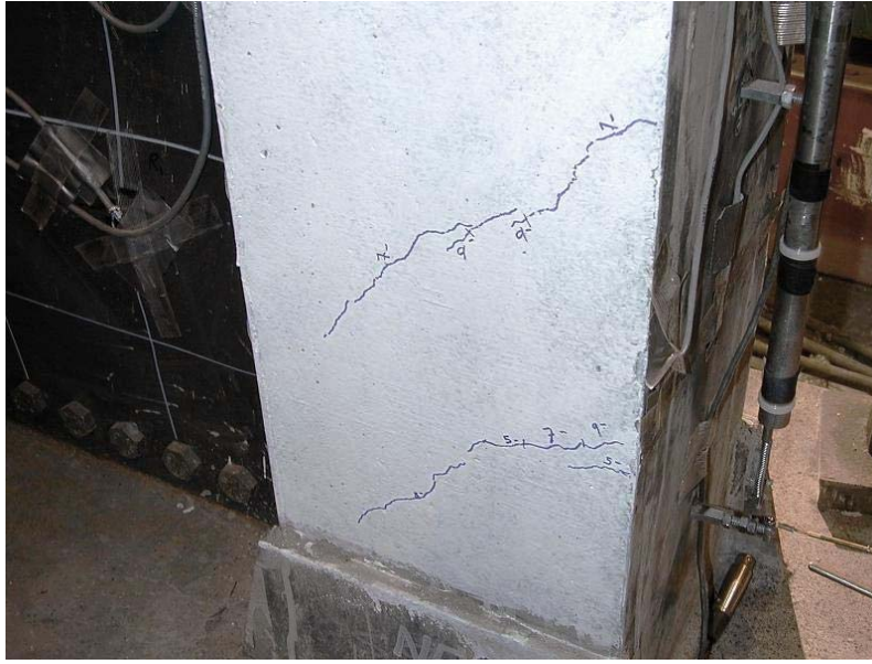
Figure 5.1: Cracks in concrete of the north PEC column in cycle 9
