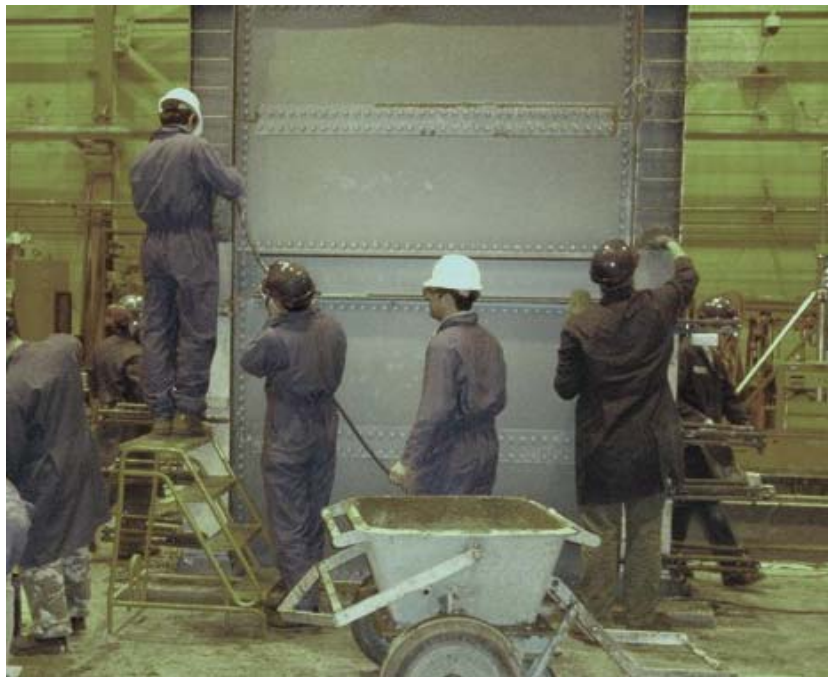
Figure 4.17: Second lift of the concrete cast in the PEC columns in the first story
