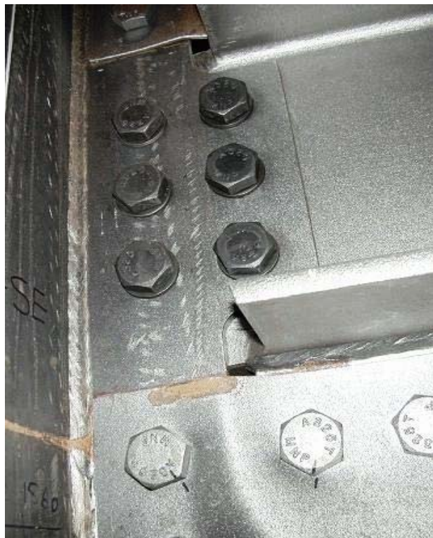
Figure 5.2: First story infill plate fold due to rotation of the frame connection
