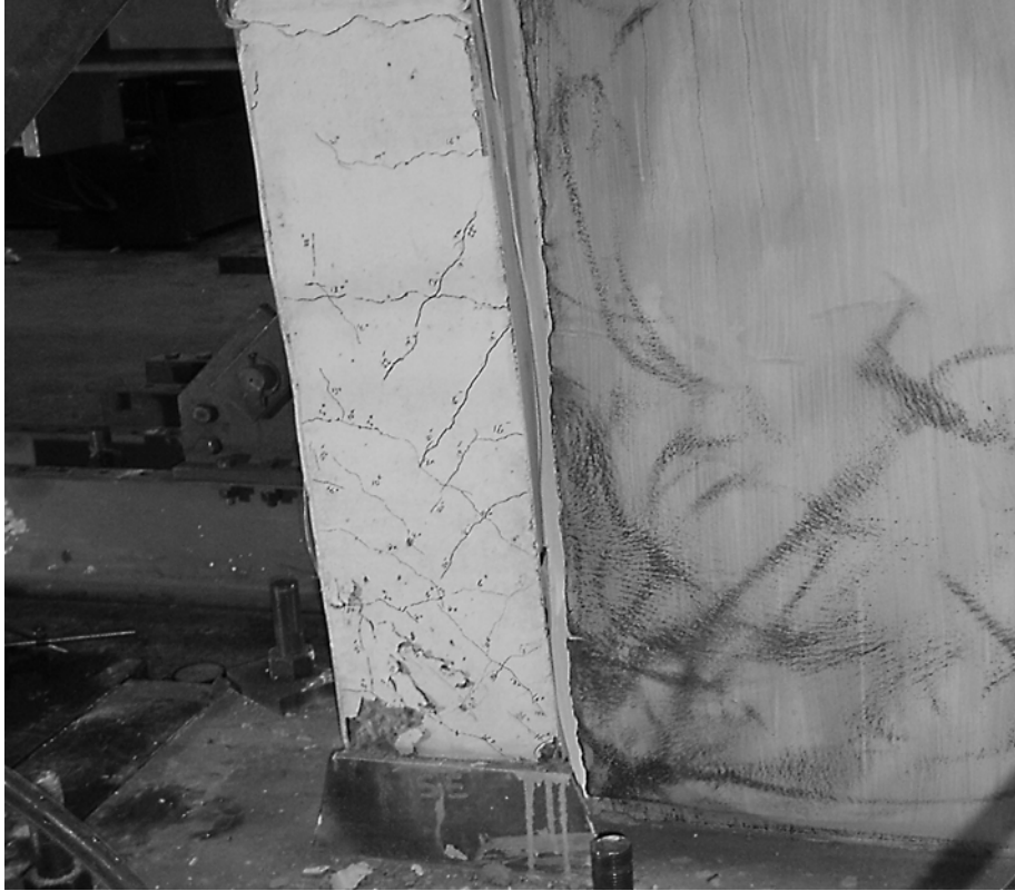
Figure 6.13: Base of the south column and adjacent infill plate, separated from the column, at the end of the test
