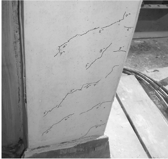
Figure 6.3: Cracks in concrete on the east face of north column in cycle 9
