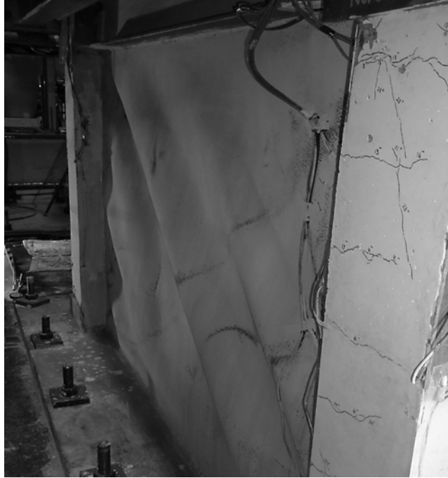
Figure 6.7: Buckled infill plate of the first story in cycle 23
