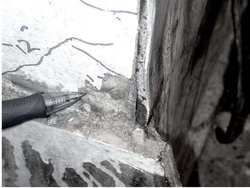
Figure 5.5: Local buckling of the outer flange just above the side plate at the base of the north column during cycle 20
