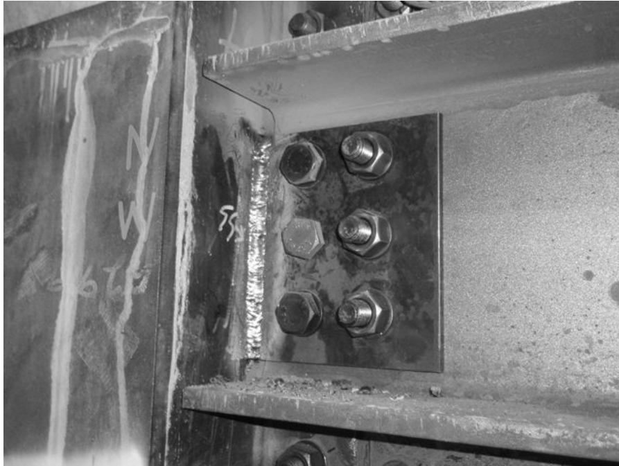
Figure 4.4: Additional fish plate in the first floor beam-to-column connection of the modular test specimen
