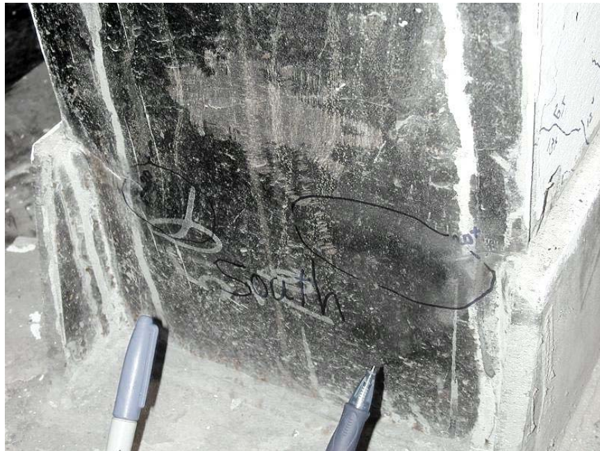
Figure 5.6: Buckling of the flange between side plates at the base of south column in cycle 20
