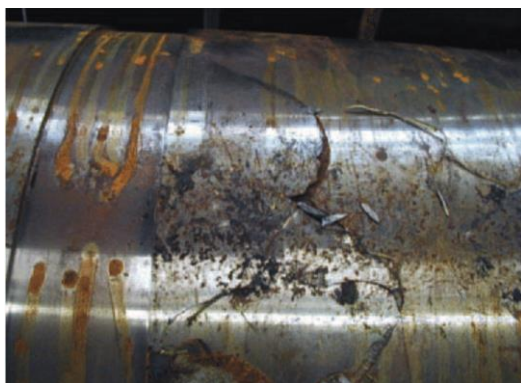
Figure 1-2 A pipeline subjected to hydrogen damage [32].
