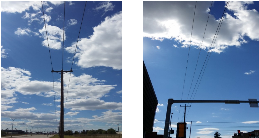
Figure 4.1: Examples of the overhead power lines that the conductors are concentrated seeing at the ground level. (Left: three-wire without neutral, right: four-wire with neutral).
