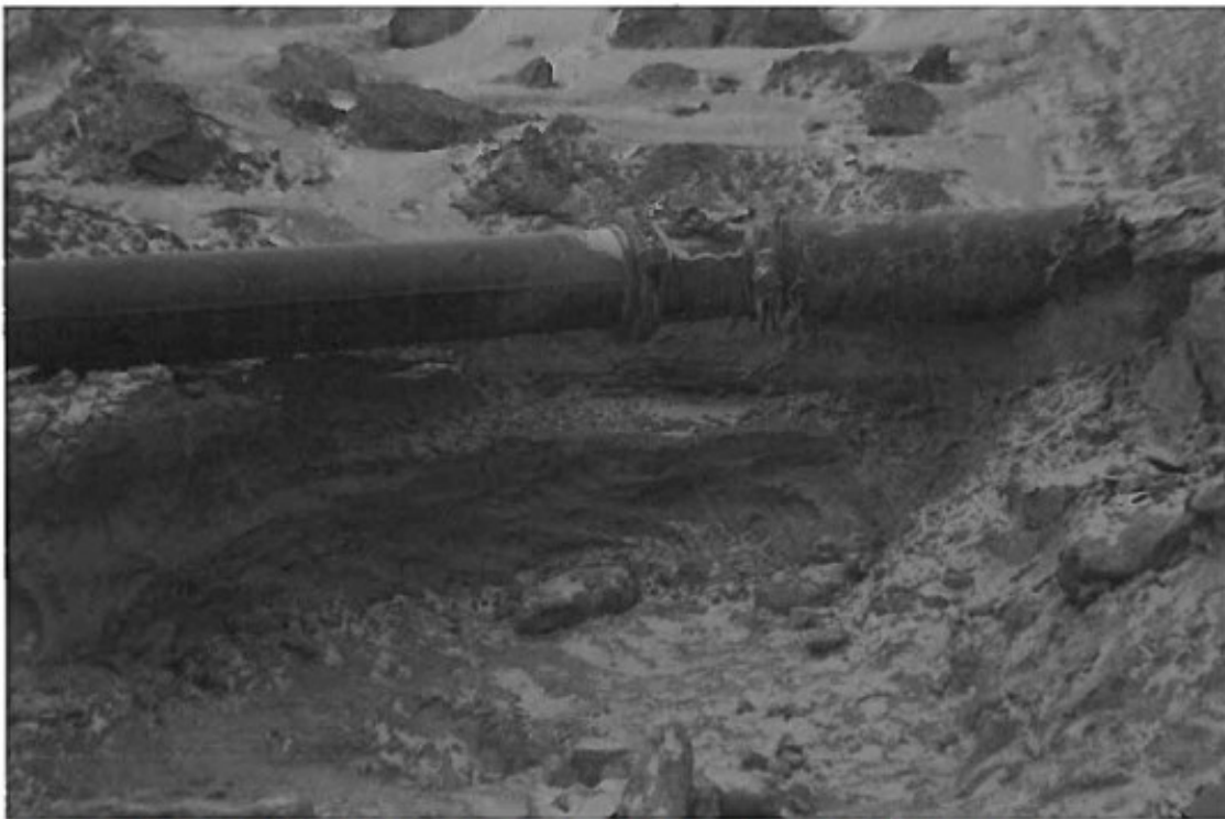
Figure 1. Location of undercut at Line 16 where the body of worker 1 was located.
