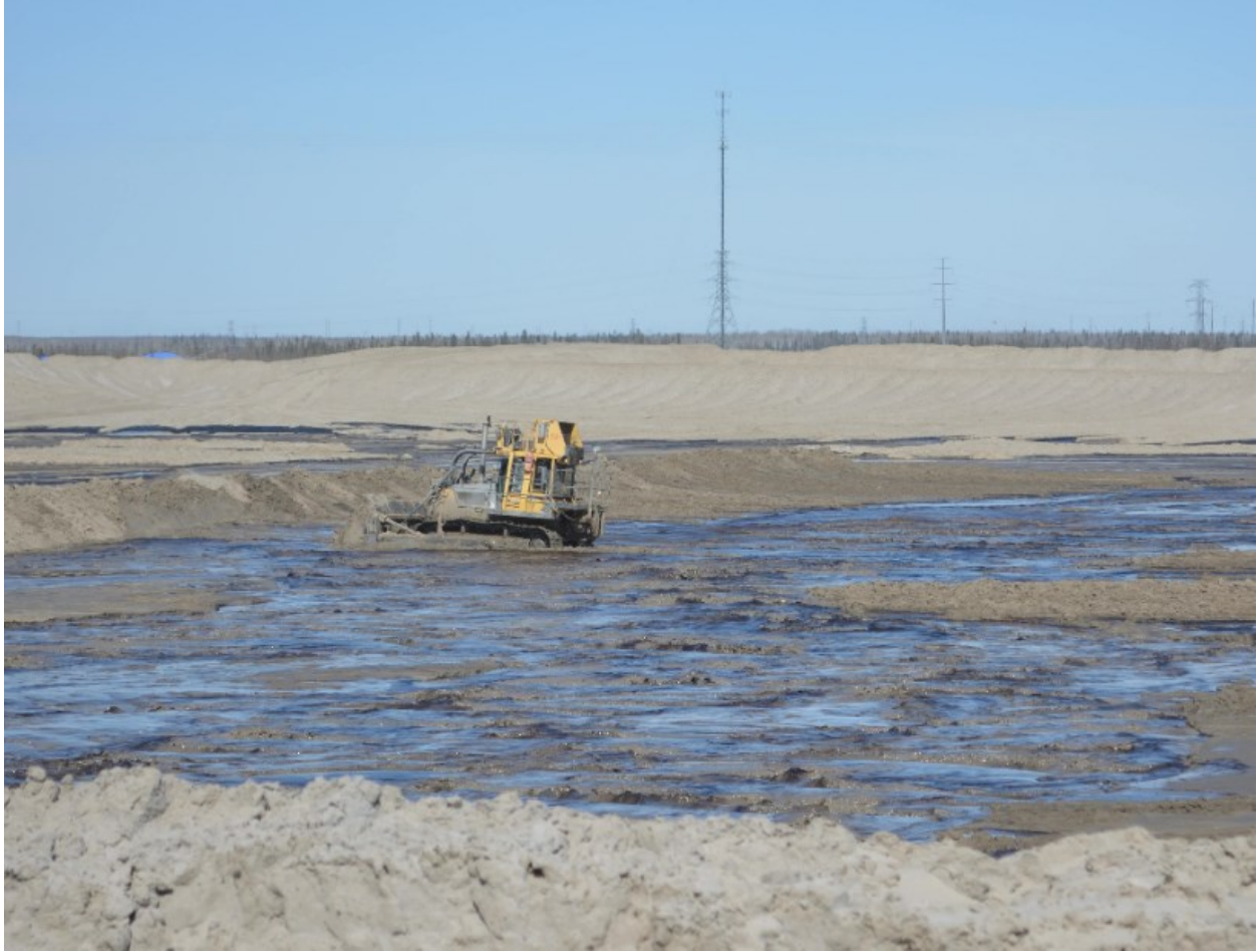
Summer Photo (e), Bulldozer working in soft ground at tailings discharge area.
