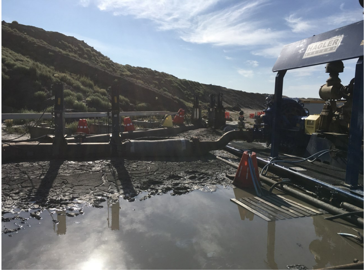
Summer Photo (d), Pumps downslope of tailings dam. Pipes and associated structures in wet, soft ground conditions adjacent to slopes
