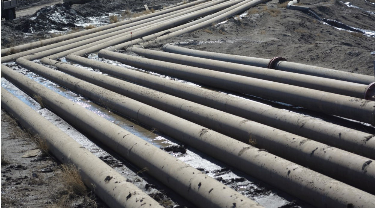
Spring Photo (f), Muddy and soft ground conditions between pipelines in working area.
