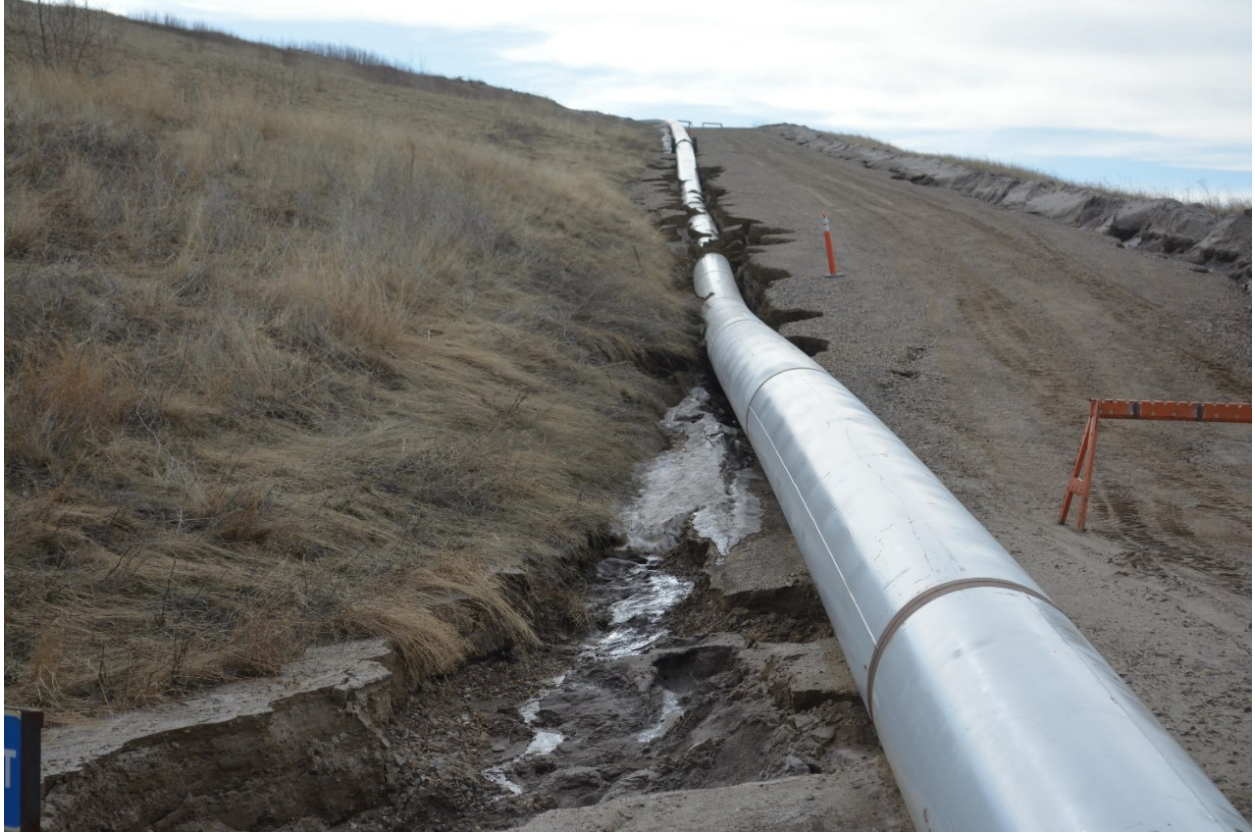
Spring Photo (h), View of pipeline that has fallen into an erosion feature next to a road.
