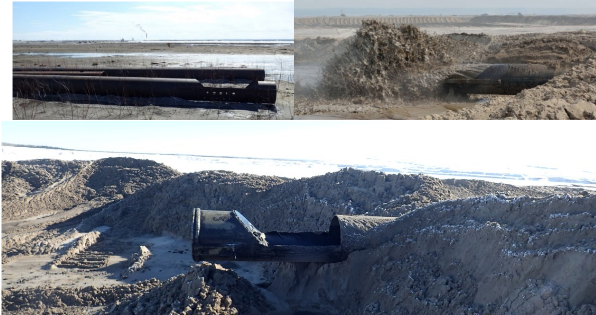
Figure 6. End of line device (or spoon): out of service (top left), in service (top right), and inactive (bottom).
