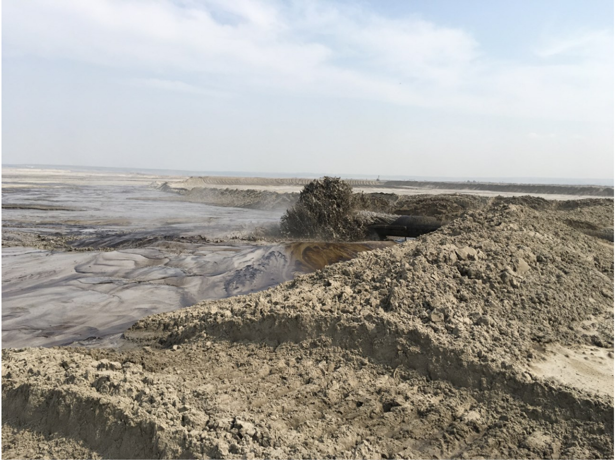
Summer Photo (c), View of tailings discharge area and end of line device (dissipates kinetic energy).
