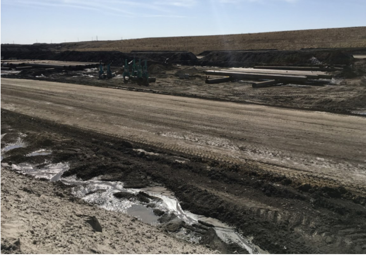
Spring Photo (c), Water ponding (right) at the toe of loose sand.
