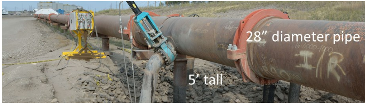
Figure 9. Photo of main line pipe.
