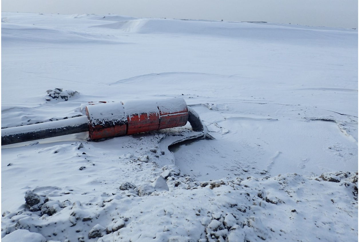
Winter Photo (f), Frozen sump pump station.
