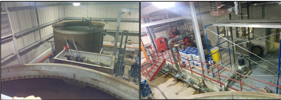
Photo 2.4.2.2. Water Treatment Plant: Storage Tanks and Machinery/Equipment.
