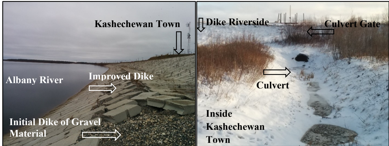
Photo 2.4.2.1. The Deteriorating Dike and a Culvert and its Gate.
