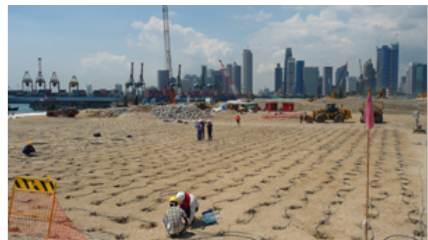
Figure 14. BeauDrain-S from the surface with lines connecting the single drains
