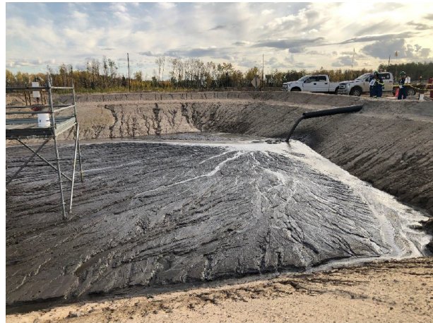
Figure 8. View of the tailings pour in Cell 2. Evenly distributed channeling can be observed.
