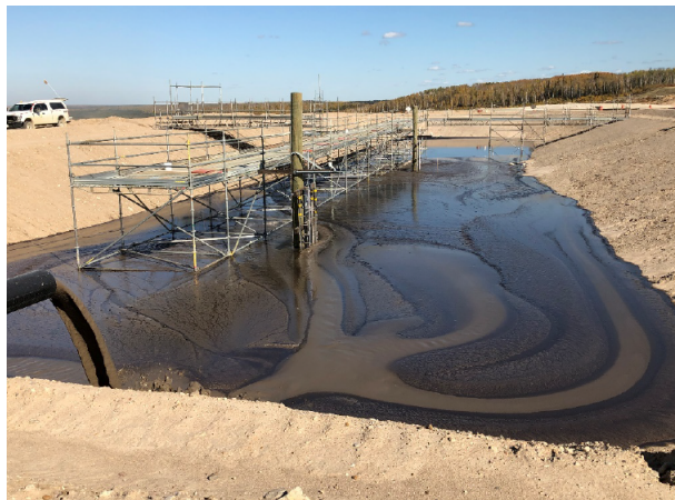
Figure 6. View of the tailings pour in Cell 1. Dominant channeling can be observed on the South side of the cell.
