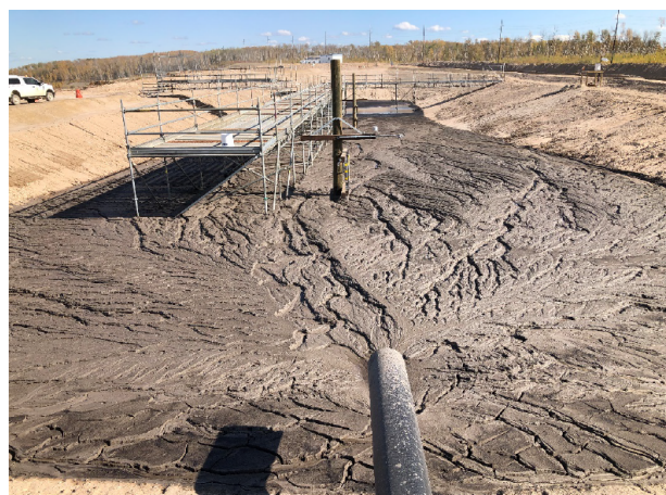
Figure 9. View of the East Cell approximately 15 hrs after cease of pour operations.
