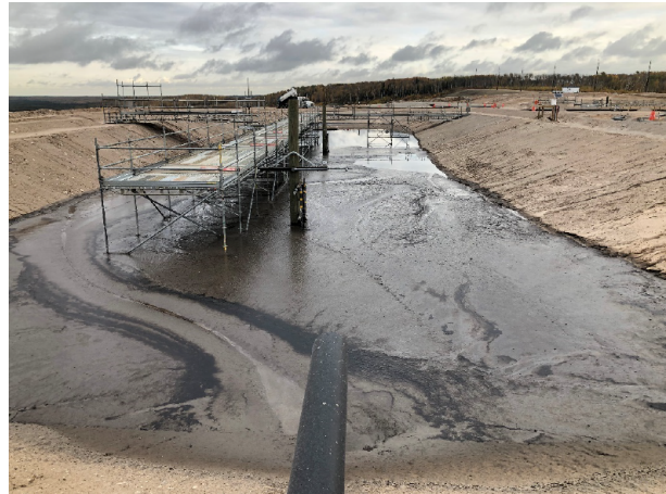
Figure 7. View of Cell 1 approximately 15 hours after ceasing pour operations. Surface of the deposit looks wet and stains of bitumen delineate the erosion gully.
