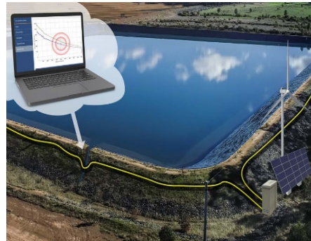
Figure 6. DTS/DBV stand-alone system for dam failure detection. Fibre optic cable is trenched in critical areas within the dam.
