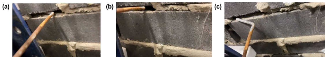
Figure C.5: T-Z.CN-2 after testing (a) connector brick interface, (b) alternative view of connector brick interface, (c) removal of connector from veneer
