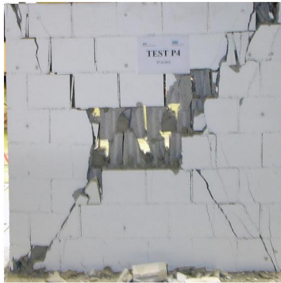
Figure 5-17. Failure mode of short URM wall in the experimental study by Salmanpour (2017)
