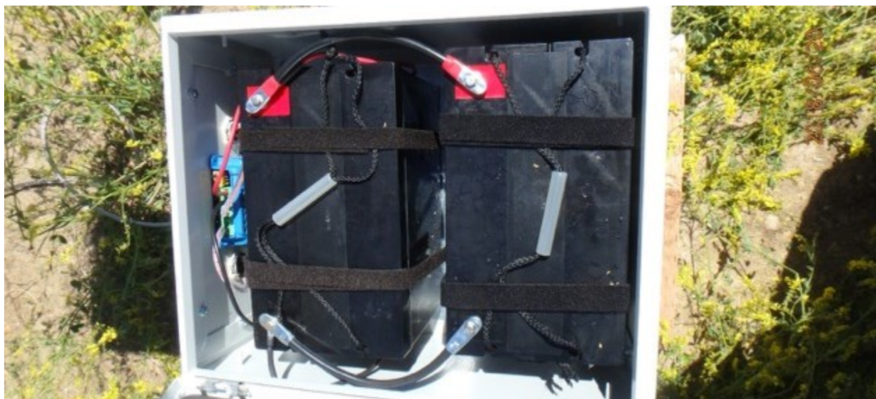
Figure 4-5: GPS battery box and batteries on Chin Coulee (Hong 2018)
