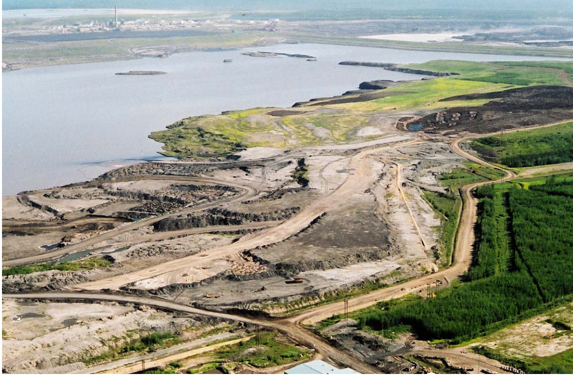
Figure I-1. Aerial view of SBH (Top Right) looking northeast during the construction phase. Photo taken between 1996 – 1999.
