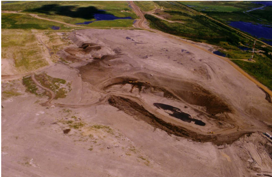
Figure I-2. Aerial view of SBH looking southeast during construction. Peat Pond was developed out of the recessed area in the middle of the photograph. Photo taken between 1996 and 1999.
