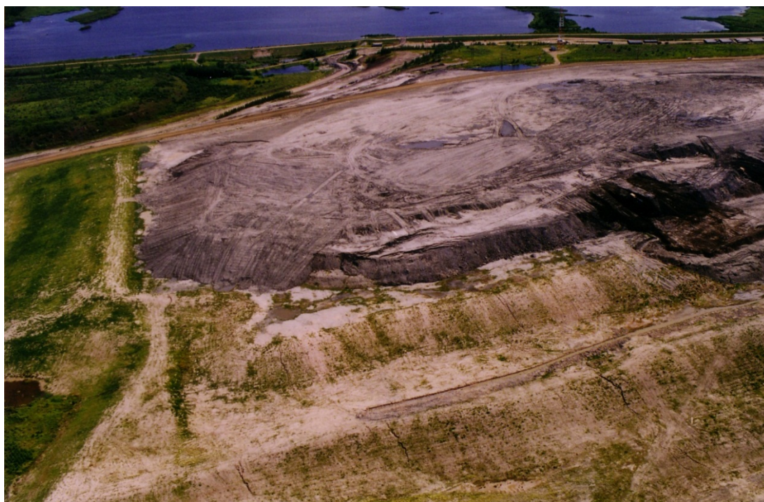
Figure 2-2. North side of SBH during regrading of upper lifts. Photo taken between 1994 and 1999.
