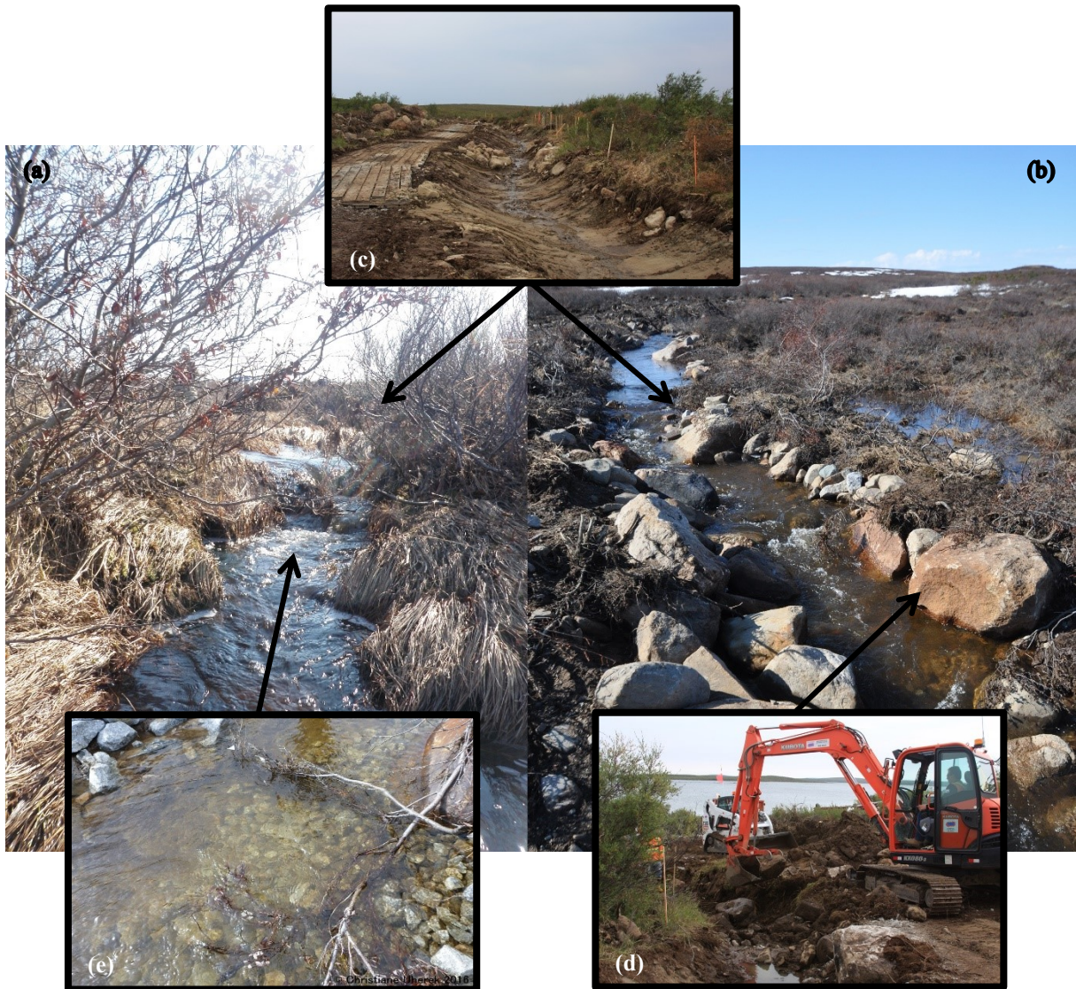
Figure 3.6: (a) West Island Stream (WIS) before manipulations; photo by M. Hulsman, taken on July 29, 2010, facing south, and (b) after manipulations; photo by C. Uherek, taken on May 31, 2013, facing south. (c) The channelization process, photo by C. Cahill, taken on August 18, 2012, facing south; (d) the boulder addition process, photo by C. Cahill, taken on August 18, 2012, facing north, and (e) wood pieces addition, photo by C. Uherek, taken on July 3, 2013, facing south.
